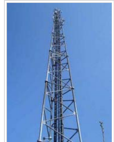
A Greenfield-type tower used in base stations for mobile telephony
